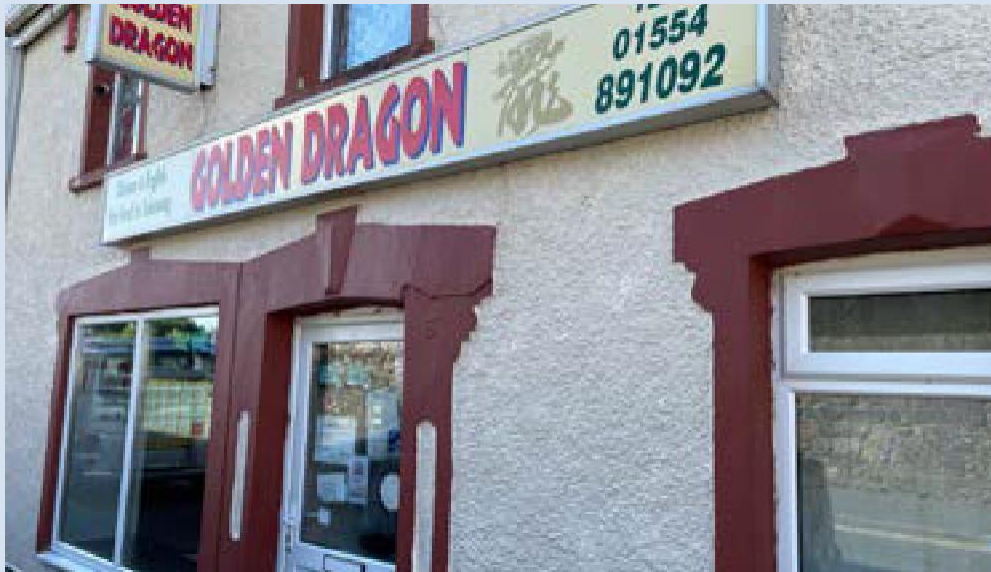
Aesthetic Value - The replacement of original details and changes to proportions can cause the original design principles of a building to be lost
